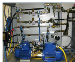
➤ HYDRAULIC CONTROL SYSTEMS
